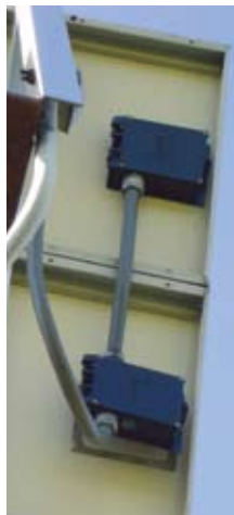
Failing double-sided junction box tape
